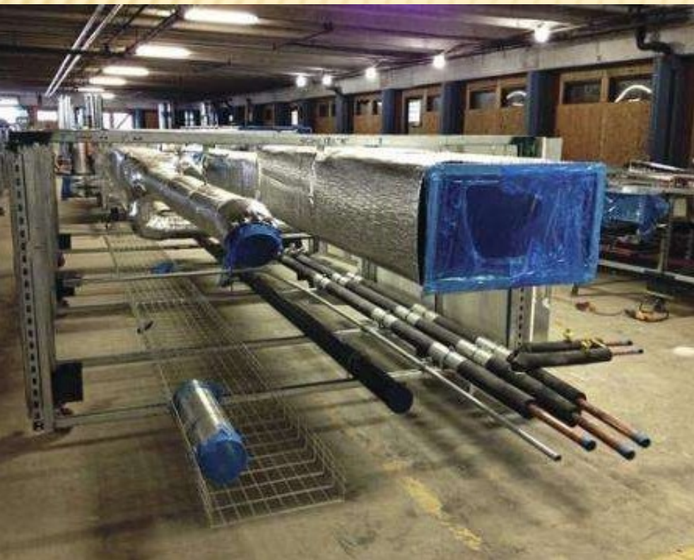
MEP Corridor Racks
